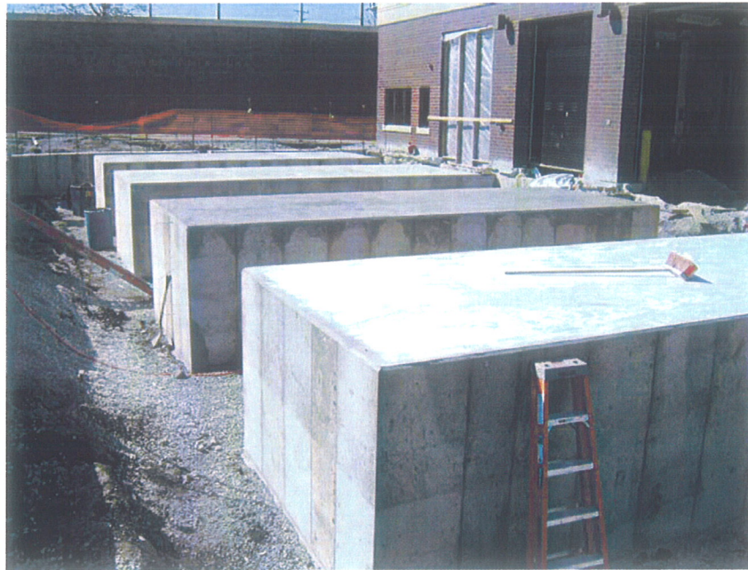
Engine-Generator Equipment Pads
