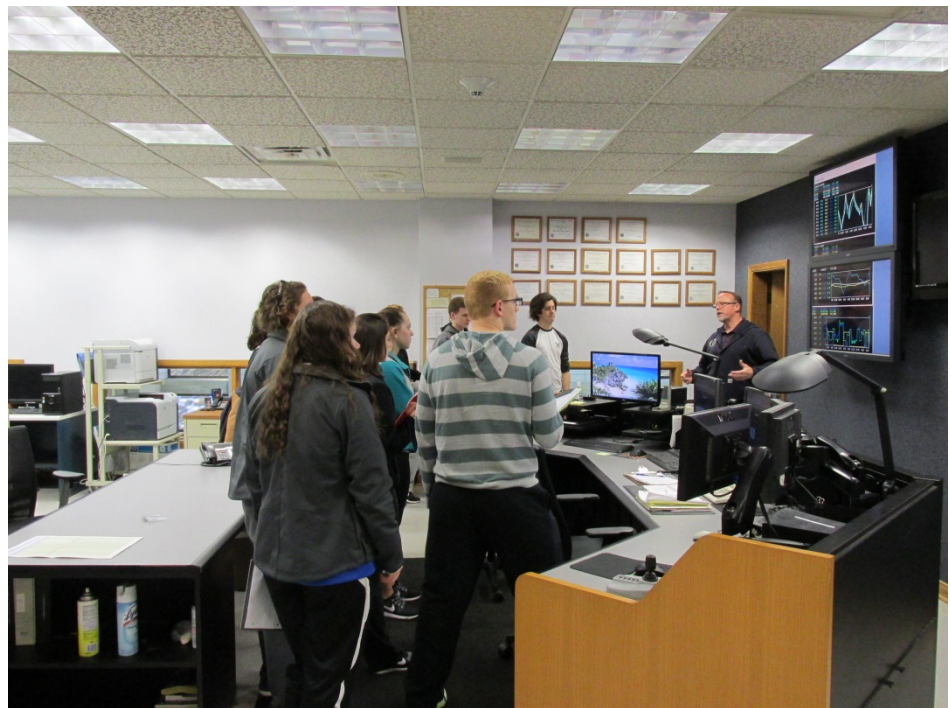
Mike Weed showing the students DWC's SCADA system in the control room
